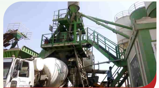
System of concrete conveyors at plants
